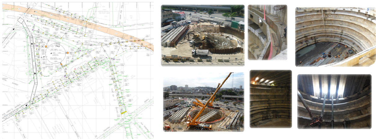
Figure 2 – Bandeira Square Detention Shaft – RT-2 - Overview of the project and photos of the building.
